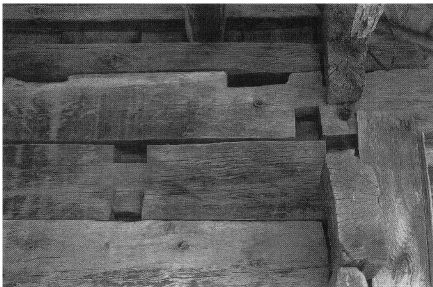
Figure 4.13. Ordu, Ünye, İkizce, Eski Cami, detail of northeast corner. Reused timbers with end dates spread out over 127 years from 1395 to 1522. (P. I. Kuniholm, ADP)
